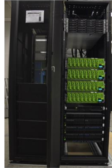
Data Core Site
